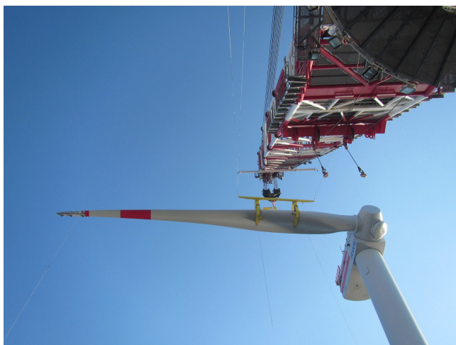
Fig. 1 Illustration of the mating phase during a single-blade installation [courtesy of RWE AG (2014)]
